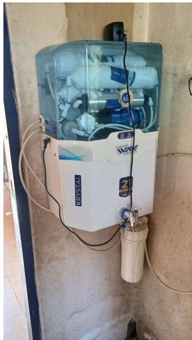
3. Drinking Water Filter unit at Kitchen of the Canteen
