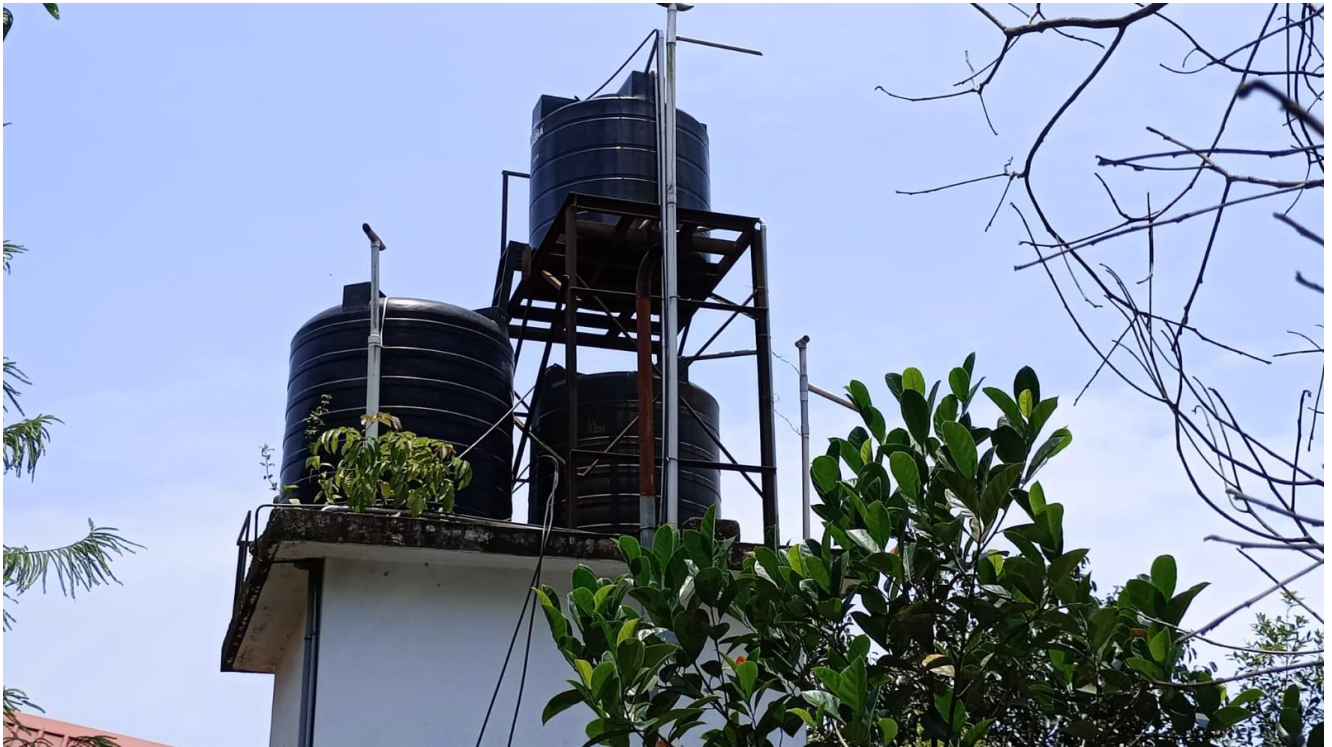
The three water tanks over the pump room
