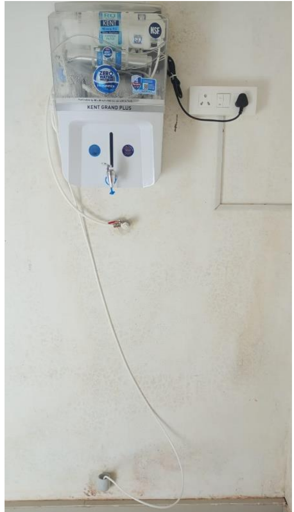
5. Drinking Water Filter unit at New Academic Block
