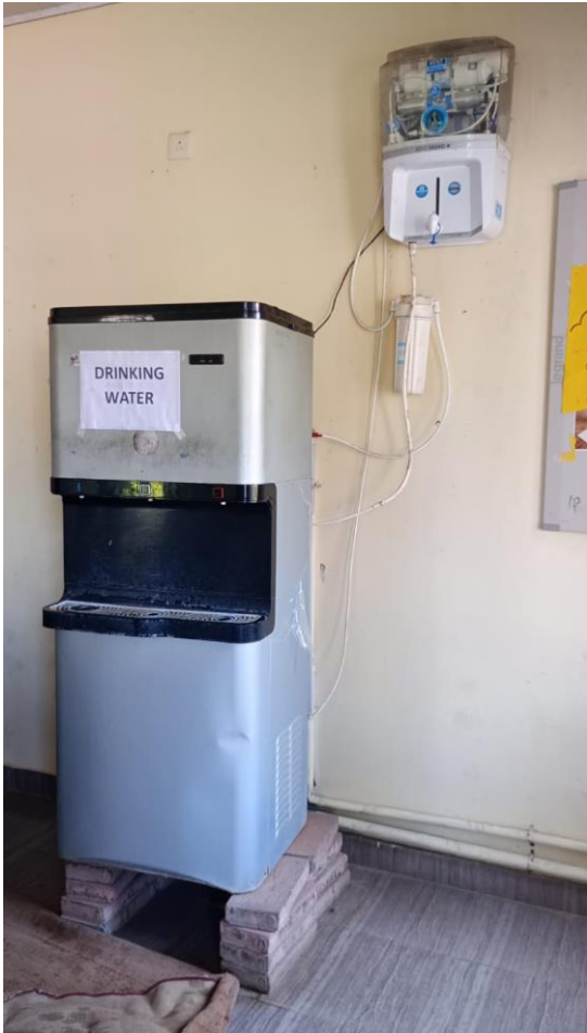
1. Drinking water filter unit in the academic block
