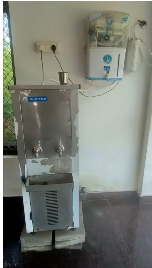
2. Drinking water filter unit in the library block
