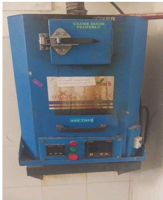
Fig 4. Sanitary pad destroying machine set up in the ladies toilet
